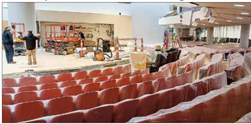
Renovation on the main assembly room of the City-County Building is underway. While construction is underway most meetings are being held next door in the small assembly room through February.
